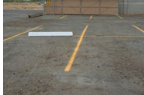
Figure 7 Employee Parking lot treated and striped with no maintenance required for 6 month period.
